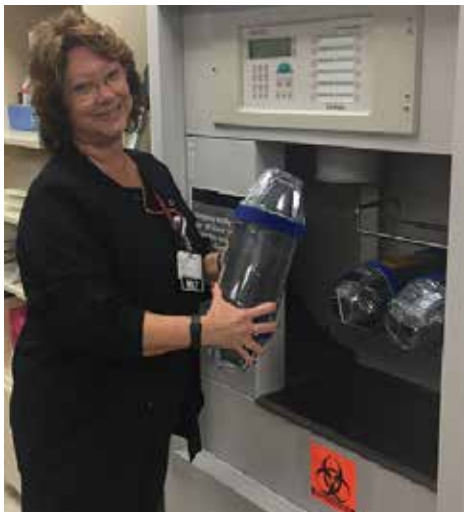
Wythe’s new pneumatic tube system allows for better lab test results turnaround time.
